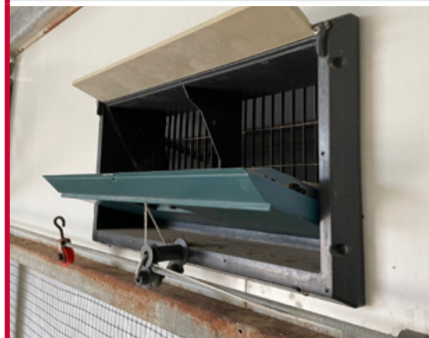
Figure 100 Example of a good-quality air inlet.
