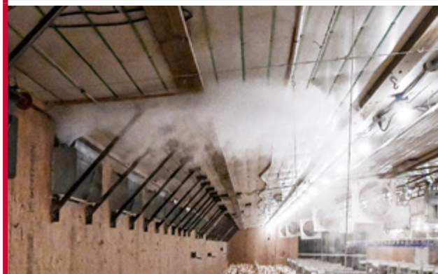
Figure 105 Using a smoke test to determine if air flow and operating pressure are correct.
