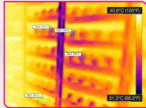
Thermal camera image of eggs chilled by faulty humidity nozzles
