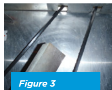
Figure 3 Worn fan belt.
